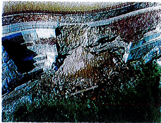
Figure 2: Slope Failure March 2022
